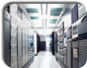
Data Center Management
